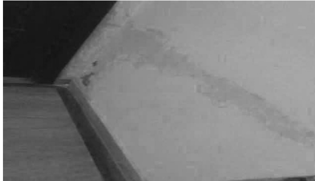
Fig. 9 Seepage on the inner walls of the house due to improper water proofing
